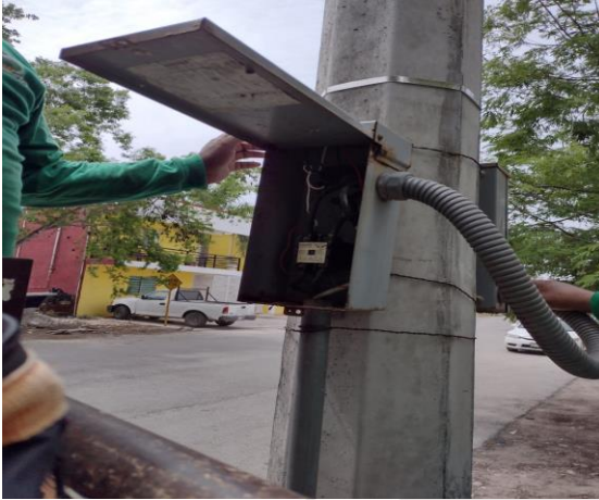
FRAC.VILLAS TULUM, C. 4 OTE / C.13, SE REHABILITA CONTACTAR PARA REPARAR SECTOR.
