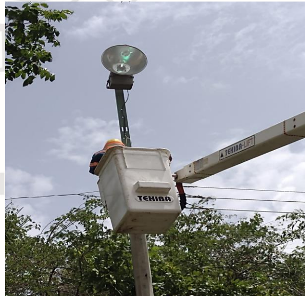
COL. TUBEN KA, C.13 M / 20 Y 24, SE REHABILITAN REFLECTORES (TIPO AM1,000W Y BALASTROS AM1,000W).
